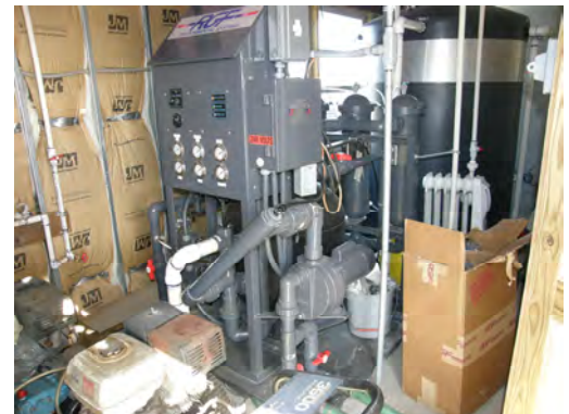
The filtration system
