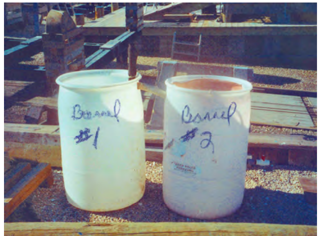
Roseman's two-barrel system facilitates the process of settling solids in wash waste water.
