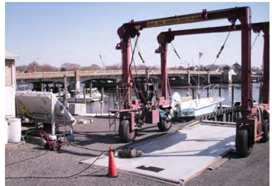
Main One's wash wastewater recycling system
