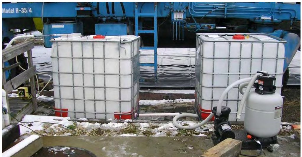
The complete wash wastewater treatment system
