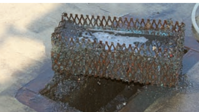
This basket captures large solids prior to the wastewater entering a 1,000-gallon settling tank.
